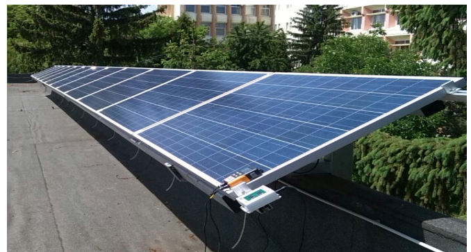
Fig. 3. The PV panels
