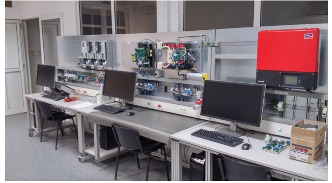
Fig. 8. The power converters systems
