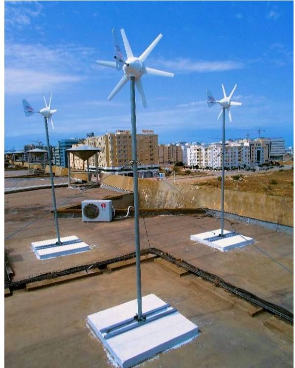
Fig. 18. Three standalone wind turbines installed above our laboratory.
